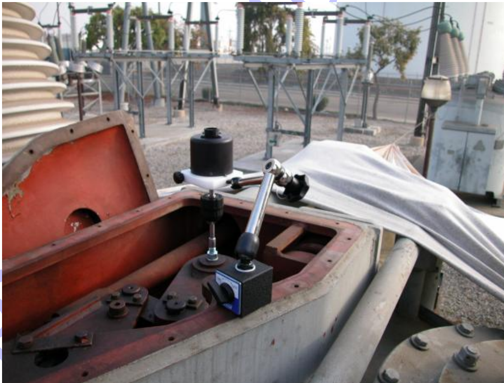
Rotary Transducer on Federal Pacific Circuit Breaker
