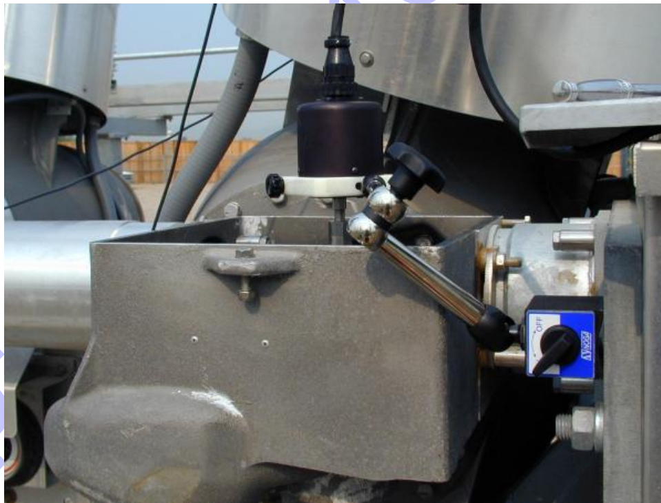
Rotary Transducer on Alstom HE 1014 Circuit Breaker
